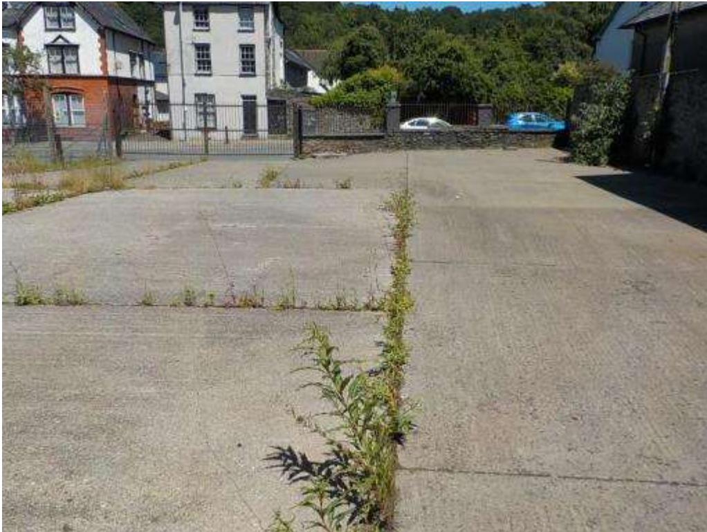
Area of hard standing at the north of the site, in front of the large shed
